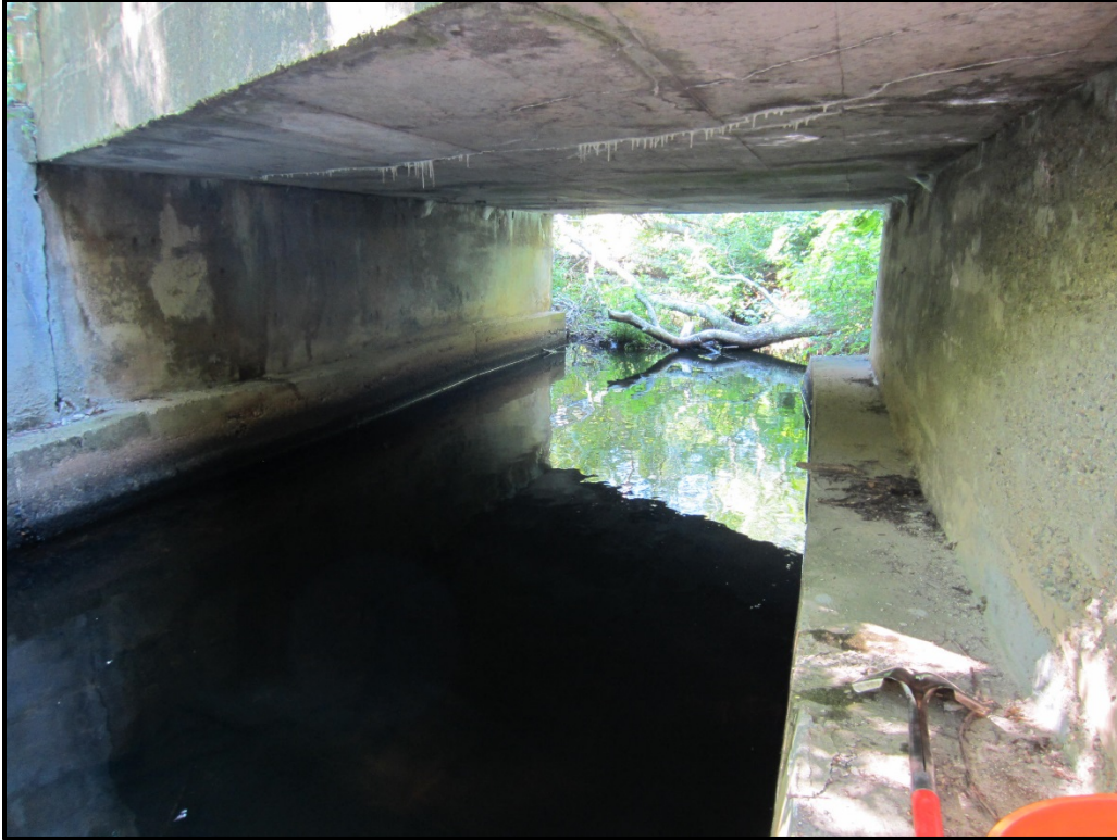
Photo 7- Looking Downstream through Bridge Opening (8/24/2016) Note Concrete Shelves both Sides
