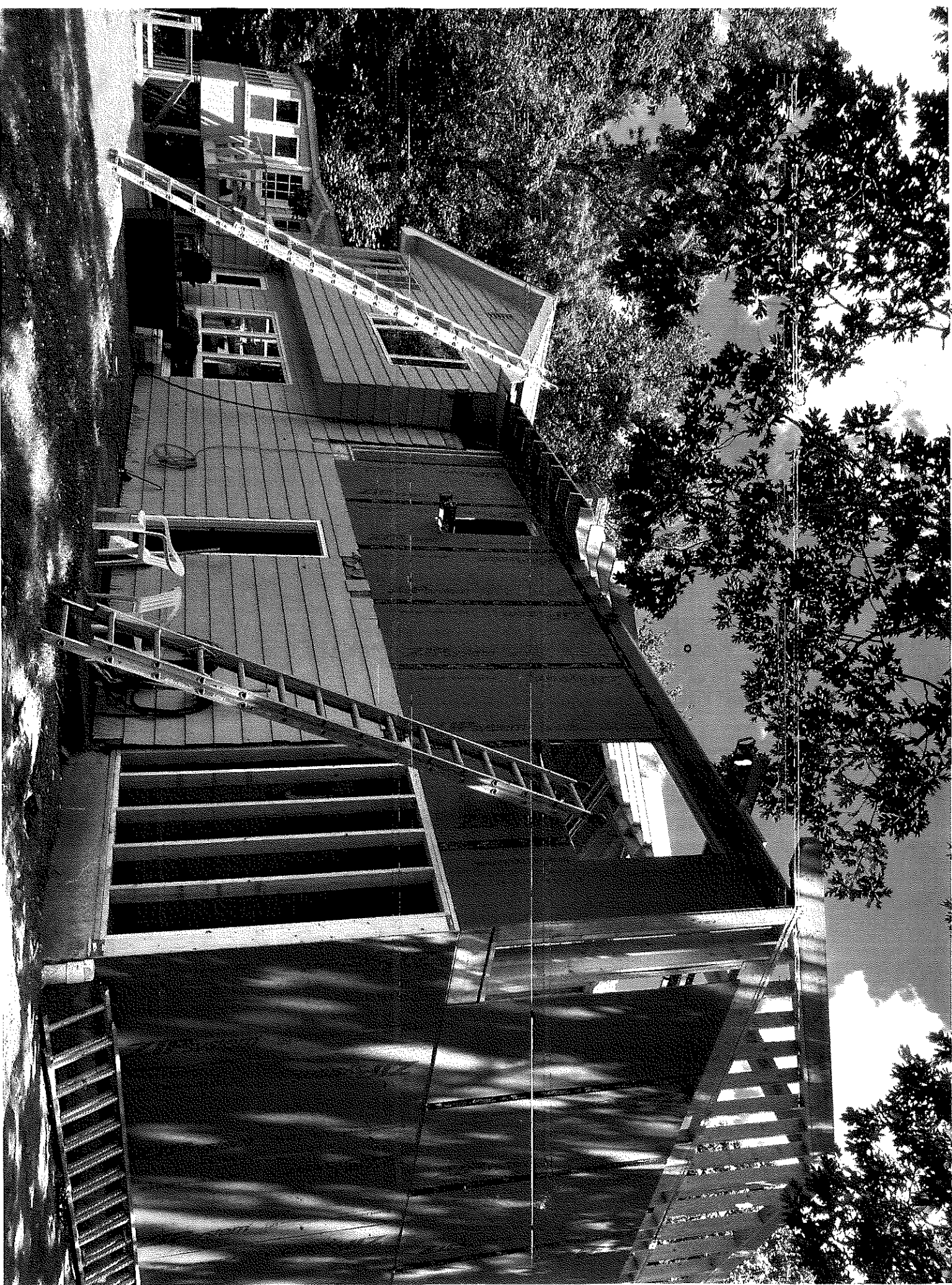
Back of Annual during Renovation (entrance to STR at opposite end, see Stowell door)
