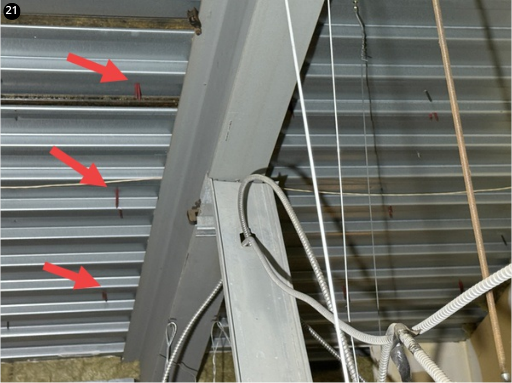
Fasteners observed penetrating deck- 11/29/24
