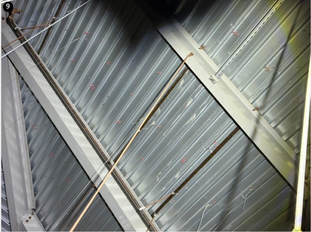
Fasteners observed penetrating deck- 11/25/24
