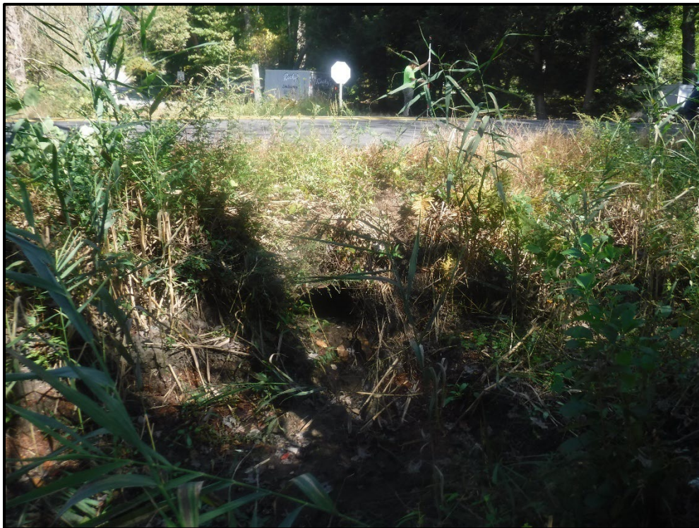
Christy Hill Road Outlet Pipe
