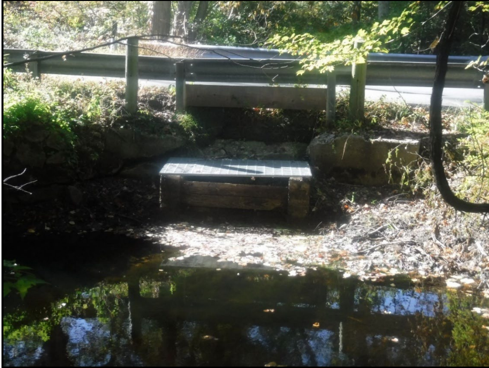
Multi-Stage Outlet Structure (Upstream)
