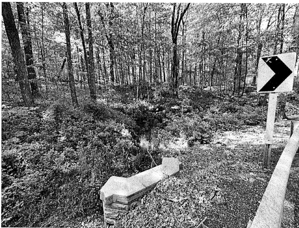
PHOTO 5: HEADWALL AT SILAS DEANE ROAD THAT INTERCEPTS FLOWS FROM WETLAND #3 AND CARRIES THE STREAM CHANNEL UNDER SILAS DEANE ROAD.
