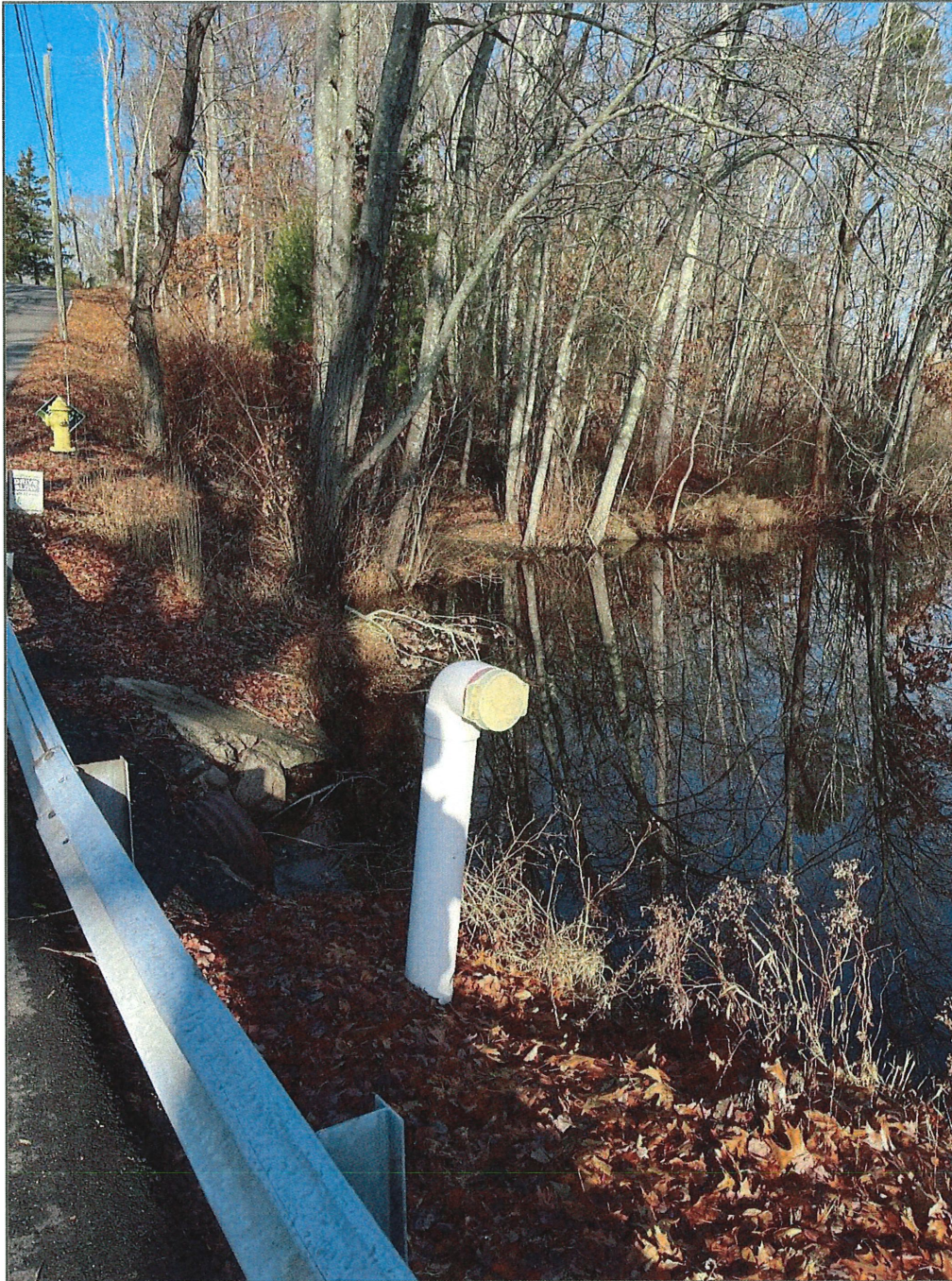
Photo 12: Dry hydrant and potable water hydrants
