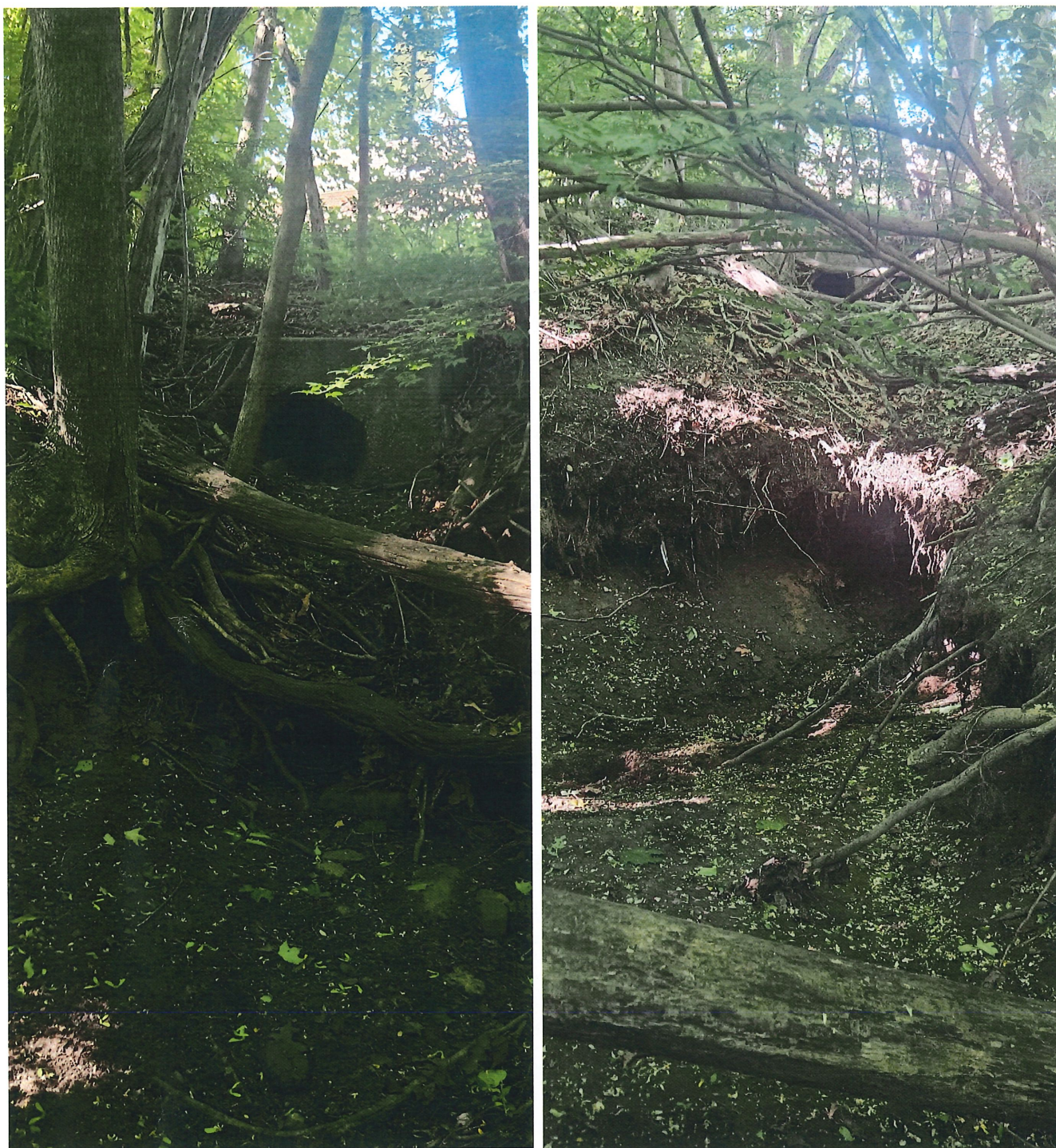
Drainage Discharge at 2 Military Hwy
