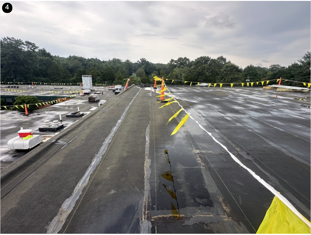
4 Water being displaced around cricket towards corner drains- Drains will be sumpt before cap sheet adhesion
