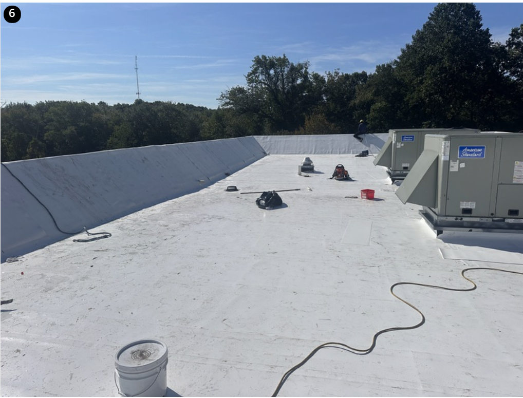
Overview- Cap sheet installed- Field seams heat welded- Curb flashings being prepared
