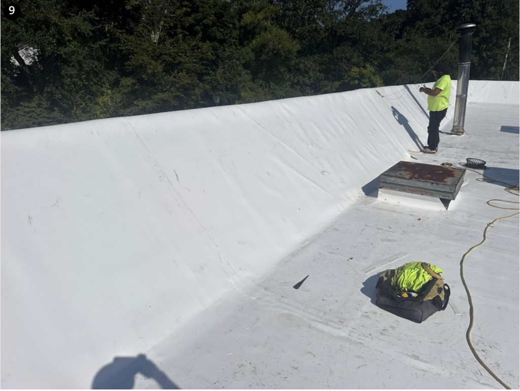
Overview- West wall near roof hatch- Roof hatch prepped for curb flashings
