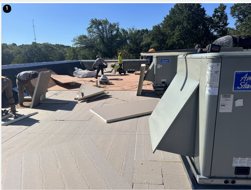
1 Crew preparing insulation boards to be adhered over mechanically fastened cover board
