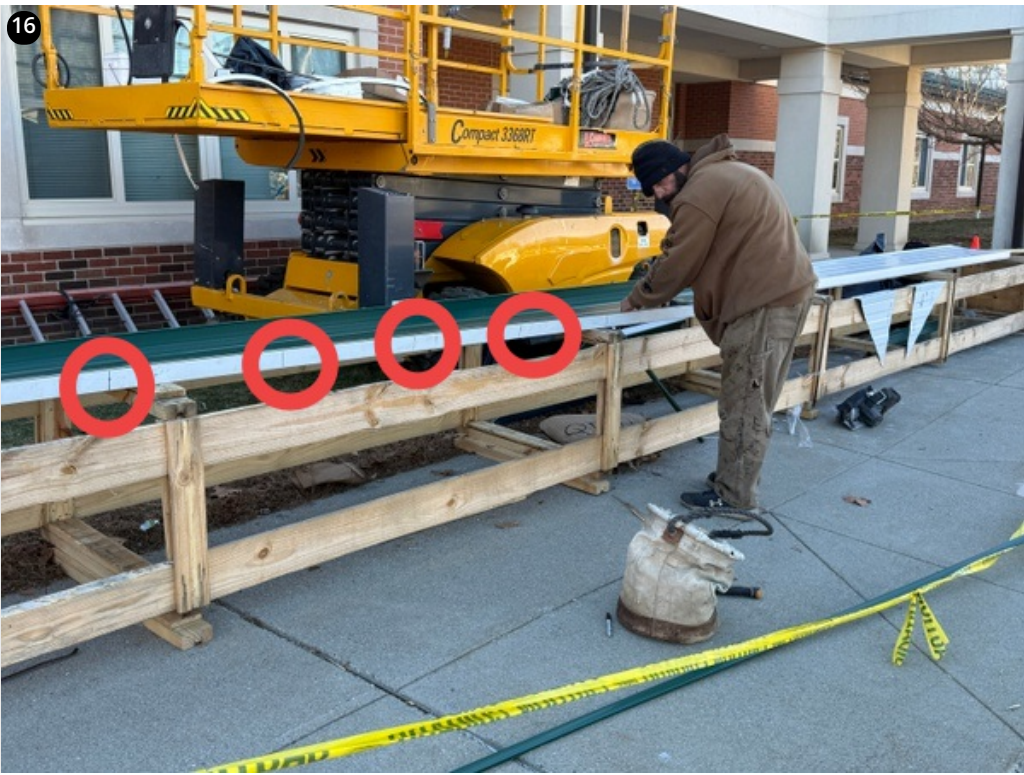
Crew marking out clip spacing per zone on panels prior to install- 11/15/24
