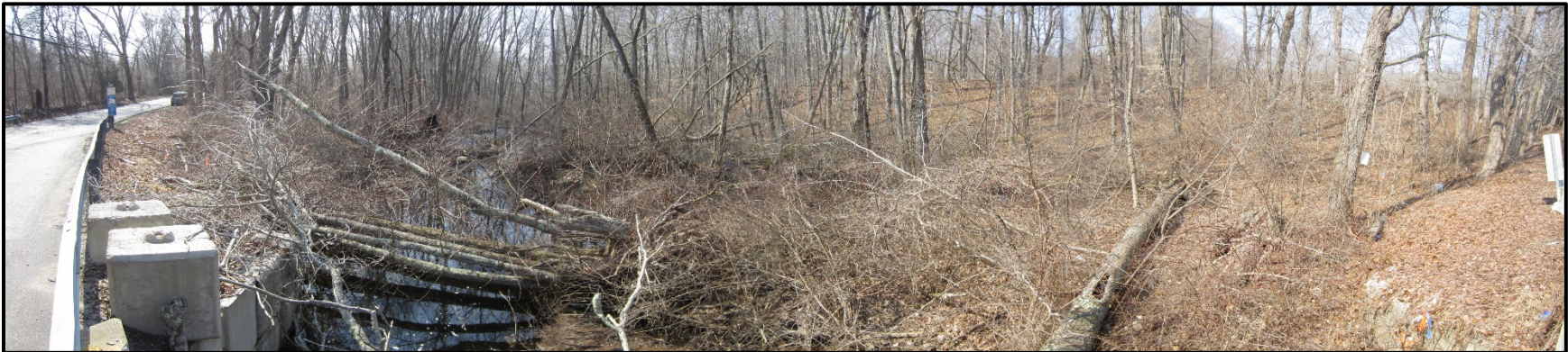
Photo 2- Looking Downstream from Bridge (3/8/2016) Note Downstream Channel Obstructions
