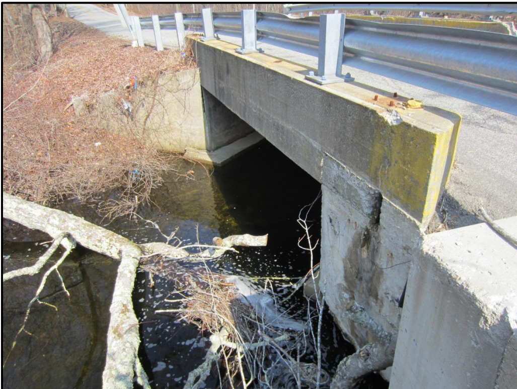
Photo 4- Downstream Bridge Face (3/8/2016) Note Downstream Channel Obstructions
