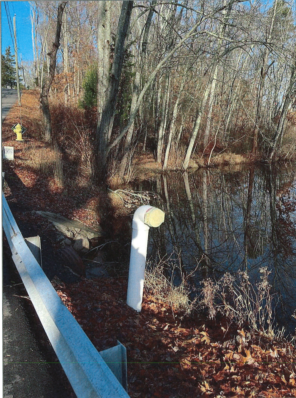
Photo 12: Dry hydrant and potable water hydrants
