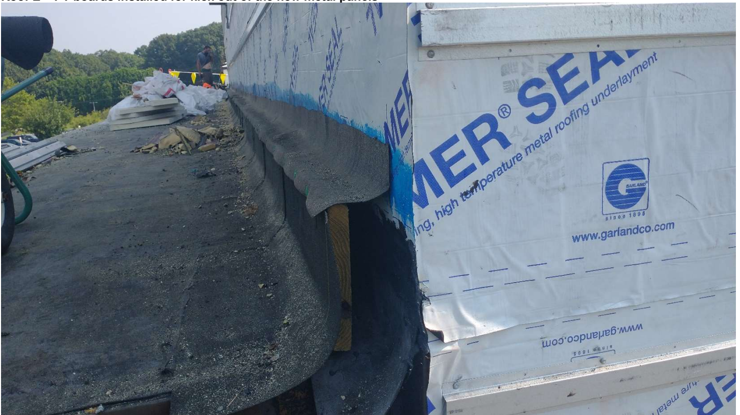
Roof E – PT boards installed for kick out of the new metal panels
