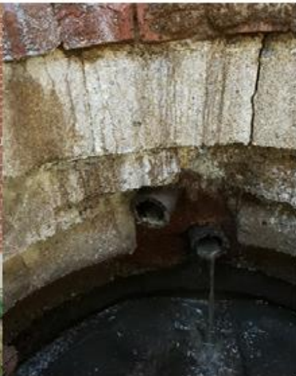
Figure 4: Force Main Discharge
