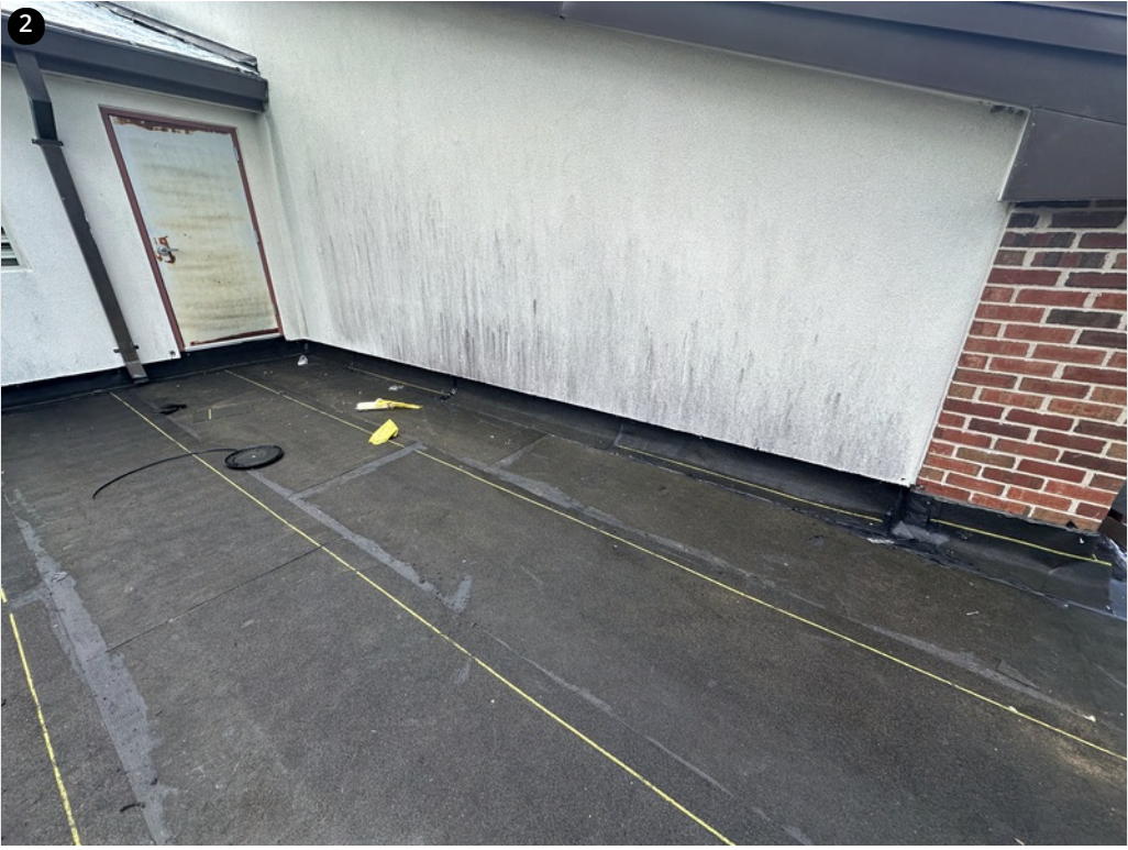
2 Completed base sheets near roof access door- Great bleedout at lap seams- Completed base flashing plys
