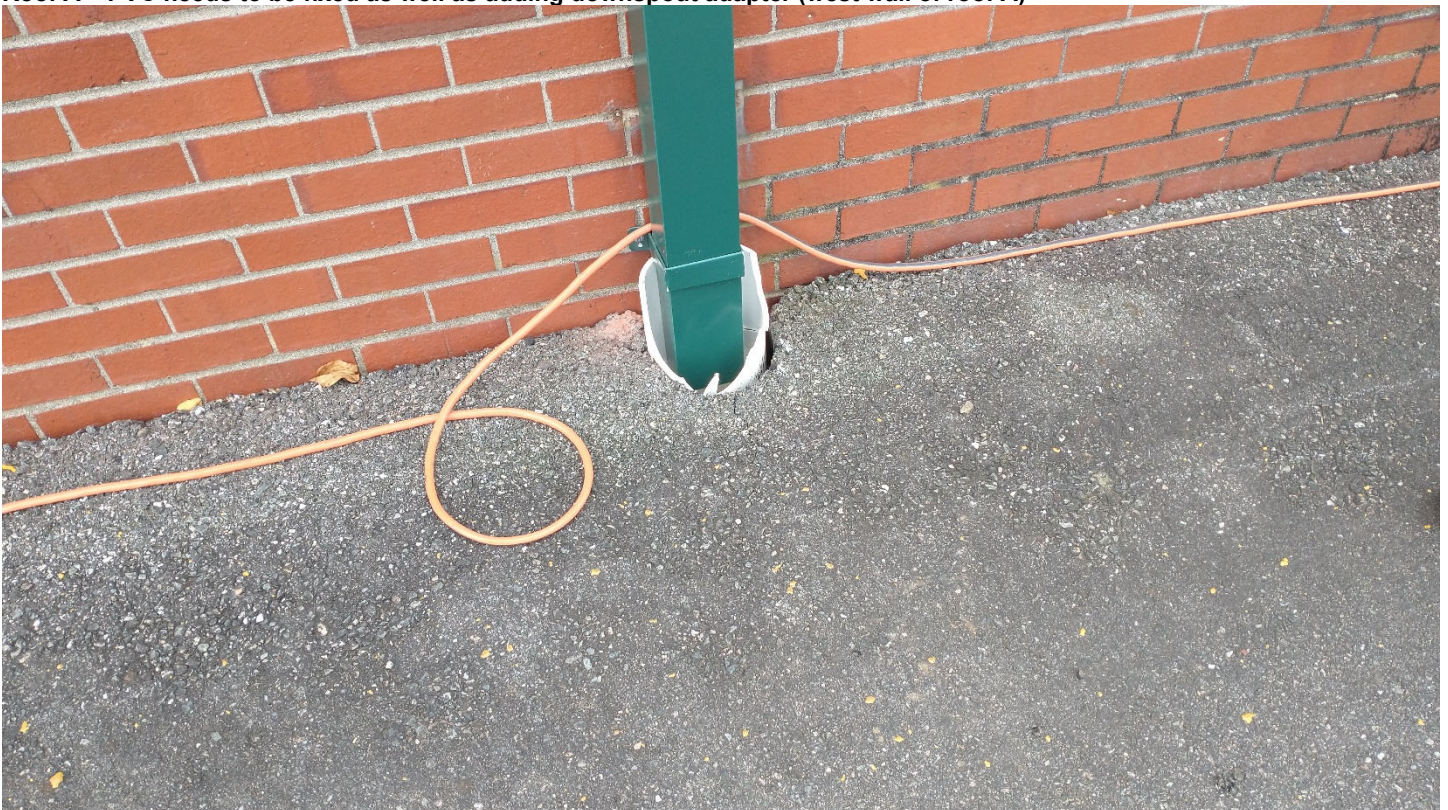
Roof A – PVC needs to be fixed as well as adding downspout adapter (west wall of roof A)
