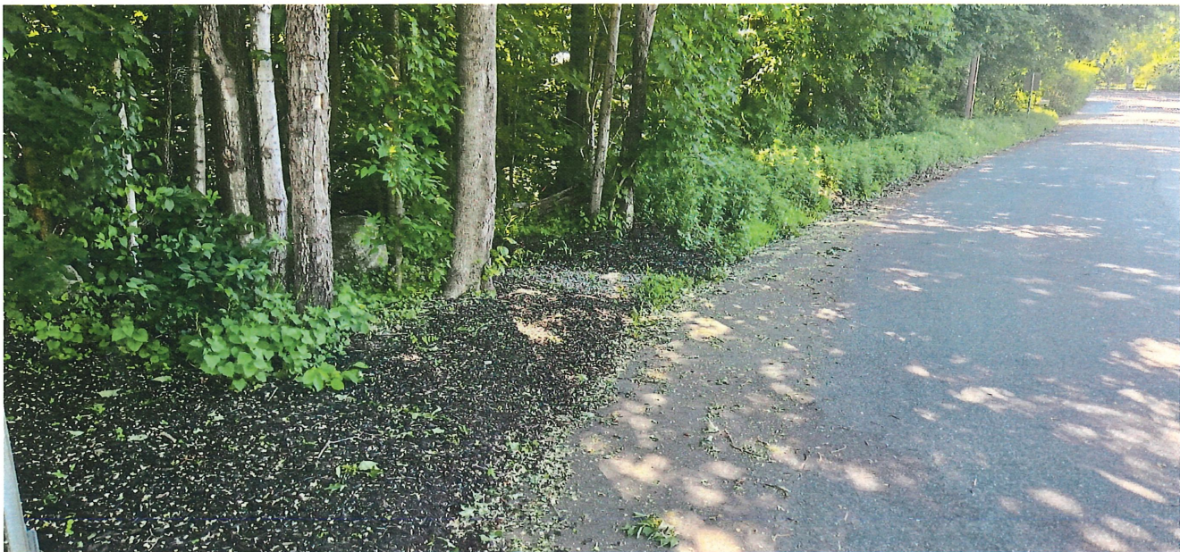
Leak-Off on to 6 Winthrop Rd west of Drainage Discharge
