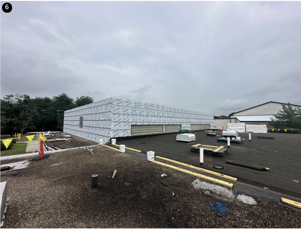
Masonry wall completely covered with ice and water- Hat channels installed
