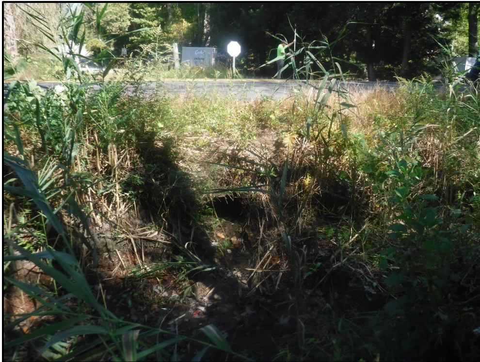
Christy Hill Road Outlet Pipe
