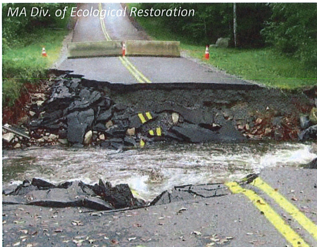
A culvert “washed out” by a storm in Beckett, MA.
