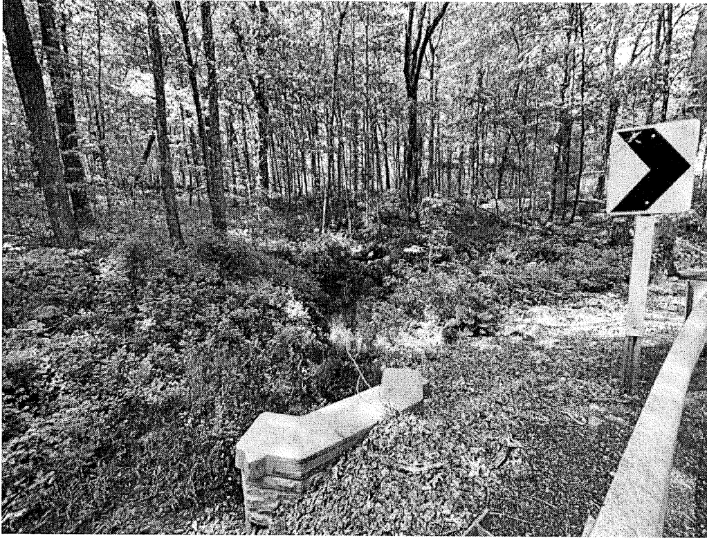
PHOTO 5: HEADWALL AT SILAS DEANE ROAD THAT INTERCEPTS FLOWS FROM WETLAND #3 AND CARRIES THE STREAM CHANNEL UNDER SILAS DEANE ROAD.
