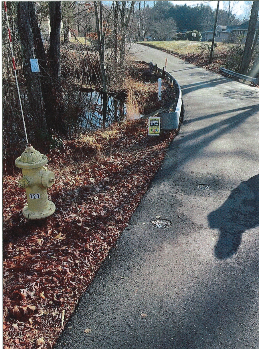
Photo 5: Water shut-off for hydrant and pipe crossing dam. Similar arrangement at left abutment
