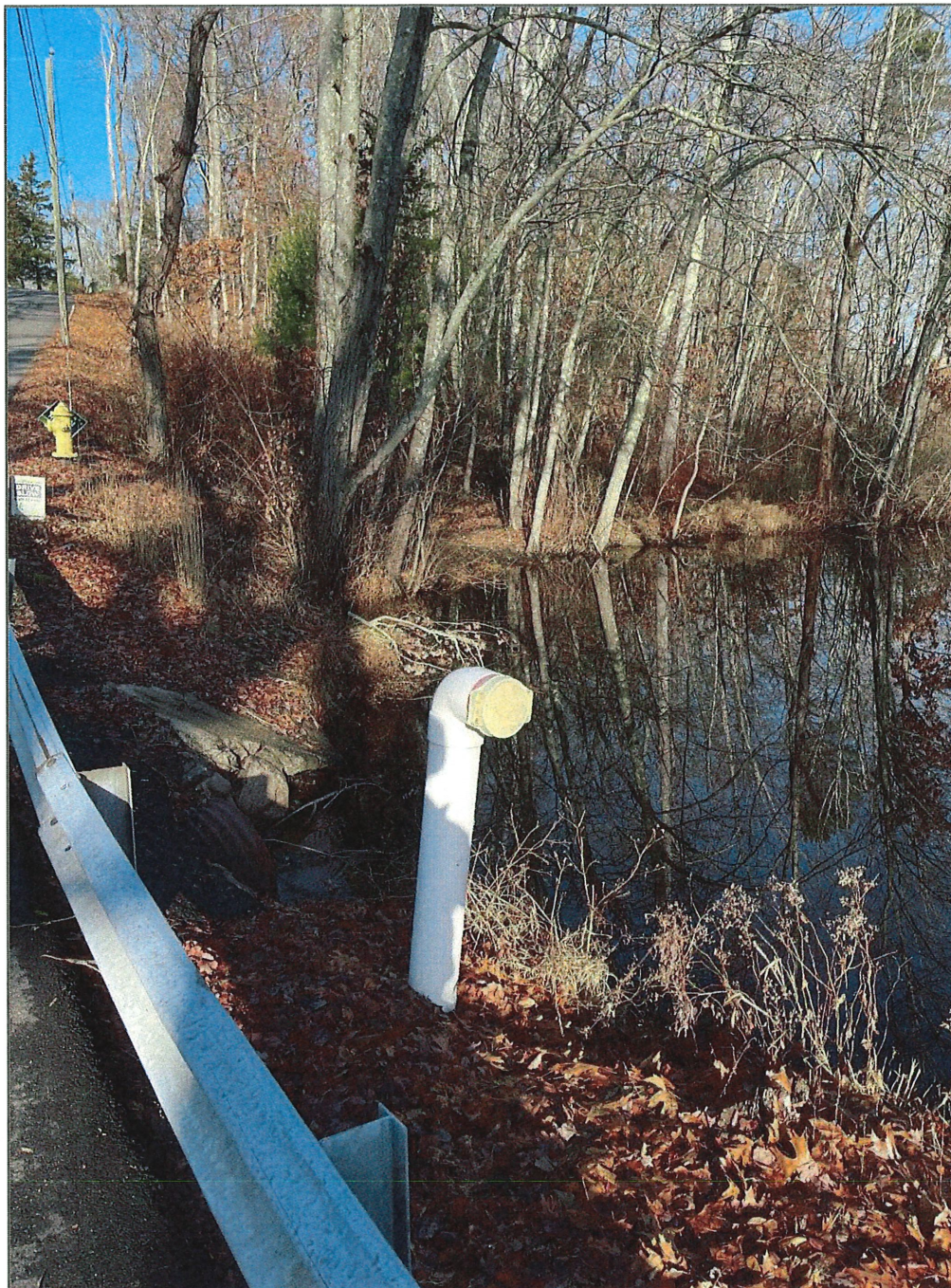
Photo 12: Dry hydrant and potable water hydrants
