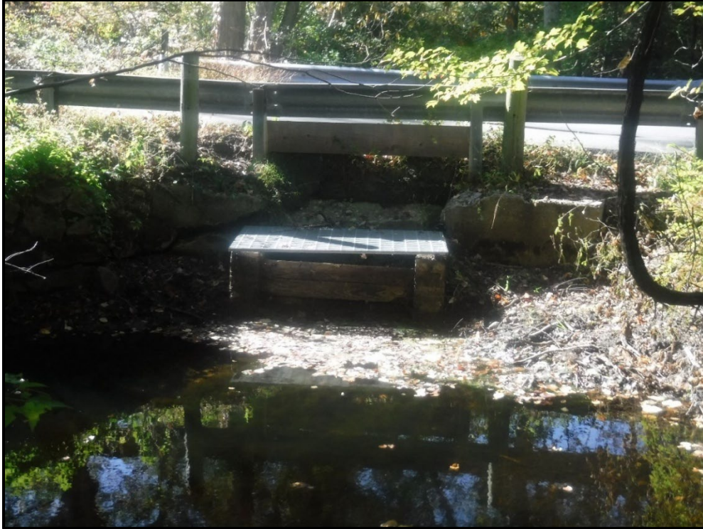
Multi-Stage Outlet Structure (Upstream)
