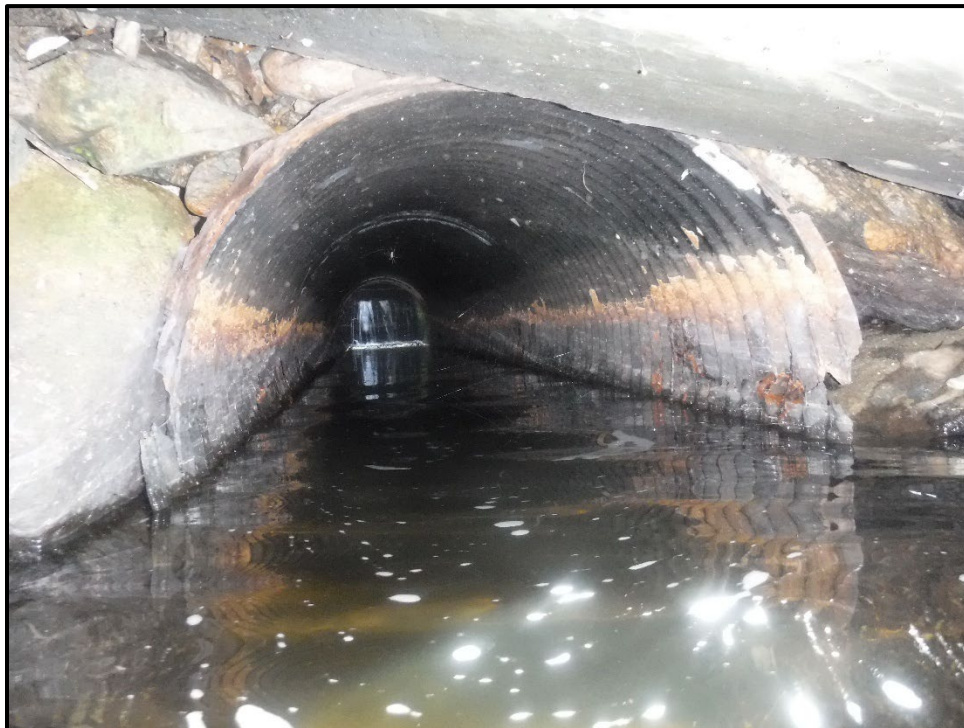
Internal Photo of 36" Culvert (Multi-Stage Outlet) with Flow Seen Penetrating Stop Boards at Head of Pipe.
