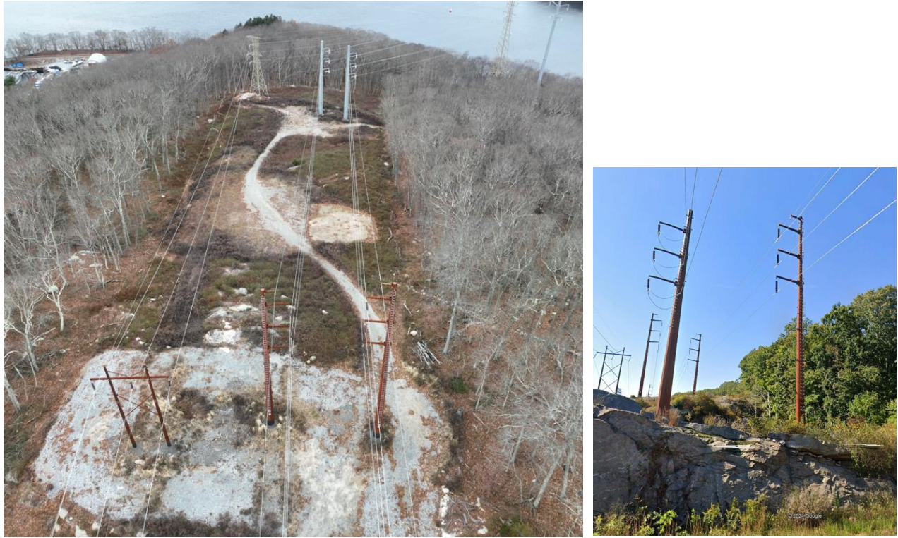
Figure 5. Eversource steel support structures adjacent to planned blasting that will take place to the right in each photograph.
