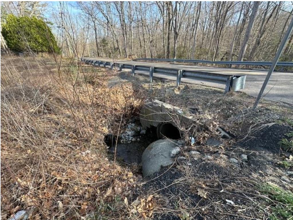
Photo 2: Failing headwall at drainage connection outlet along shoulder of Christy Hill Road.
