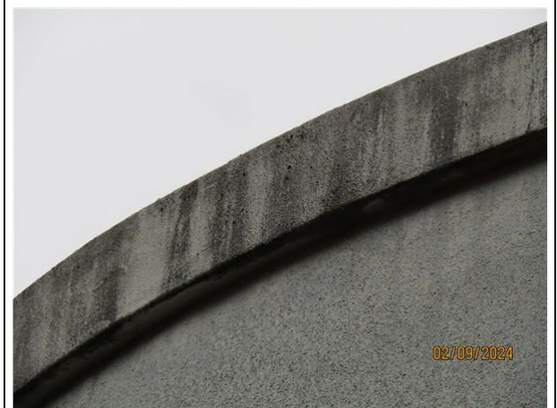
12) Biological staining along the rim of the roof
