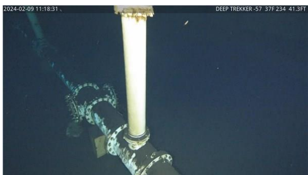
45) 14:27 - Combination inlet and outlet tree running horizontally across the tank floor
