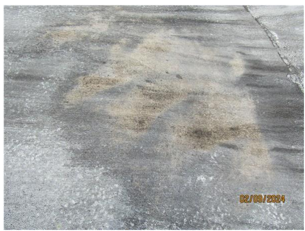
21) Area of discoloration on the exterior roof
