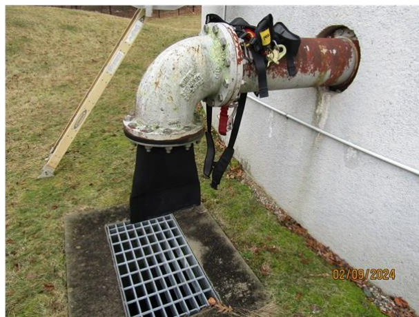
3) Overflow pipe with duck bill discharging into concrete catch basin
