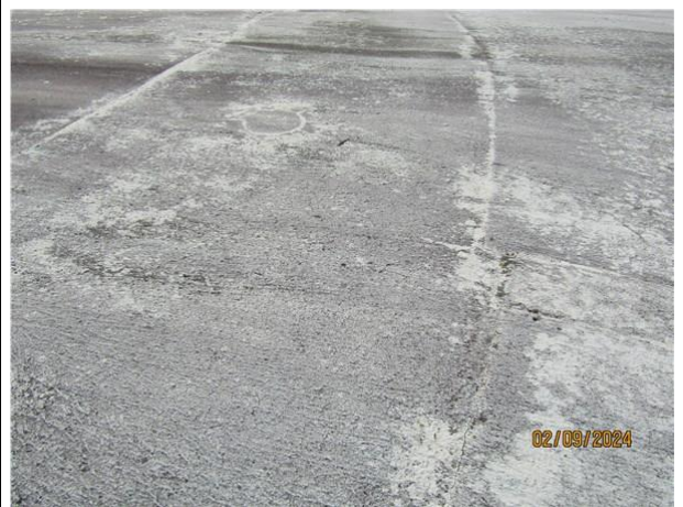
18) Weathering of exterior roof surfacing material
