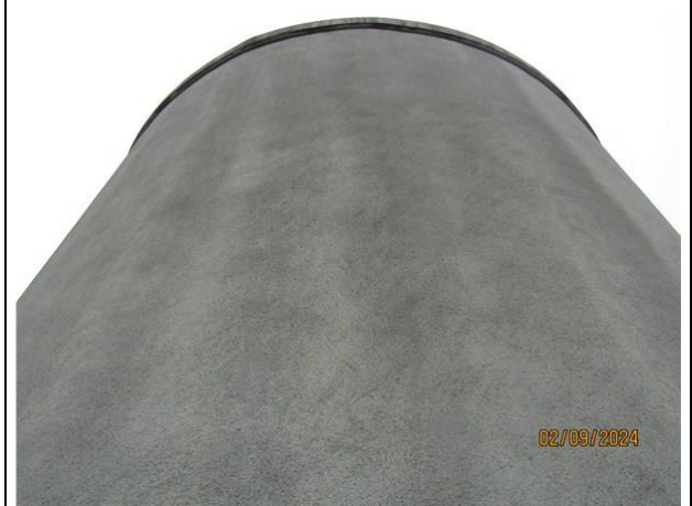
6) Typical condition of the exterior tank shell free of cracking and spalling
