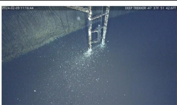
43) 12:40 - Oxidation of interior ladder due to dissimilar metals used on the safety climb
