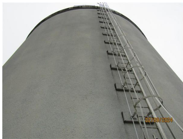
2) Shell mounted roof access ladder with safety climb and cage
