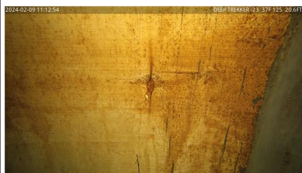
42) 8:50 - Corrosion cell from exposed rebar tie in
