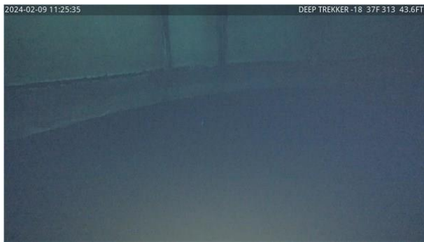
50) 21:31 - 1/4-in layer of sediment forming across the floor of the tank
