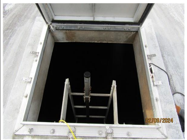
24) Interior ladder with safety climb installed under hatch
