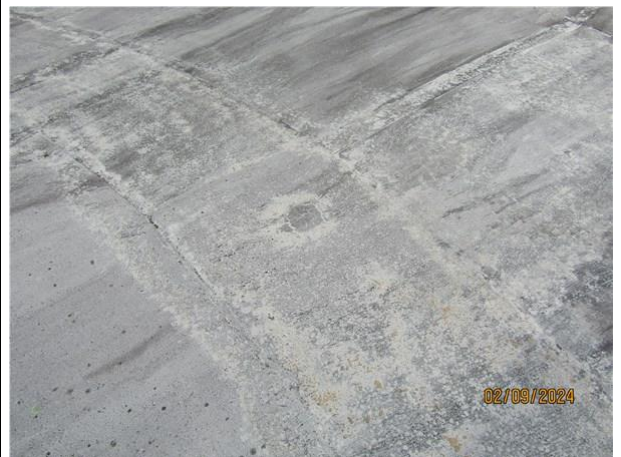
17) Biological staining of the exterior roof
