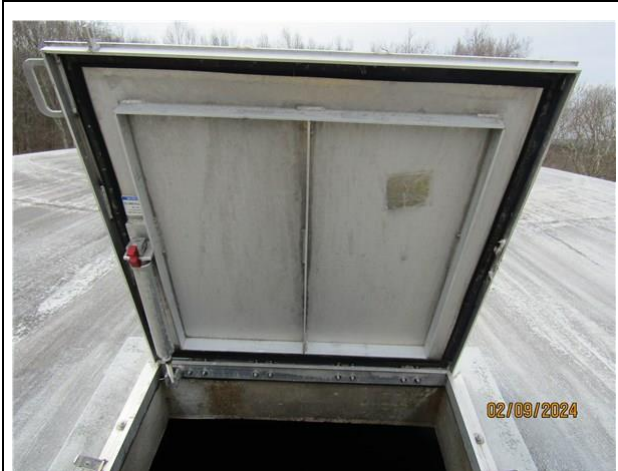
25) Intact hatch cover gasket
