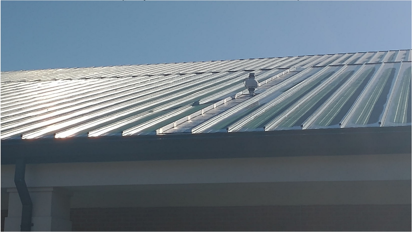
Roof A – Radon vent needs to be temporarily disconnected for the installation of the metal panels
