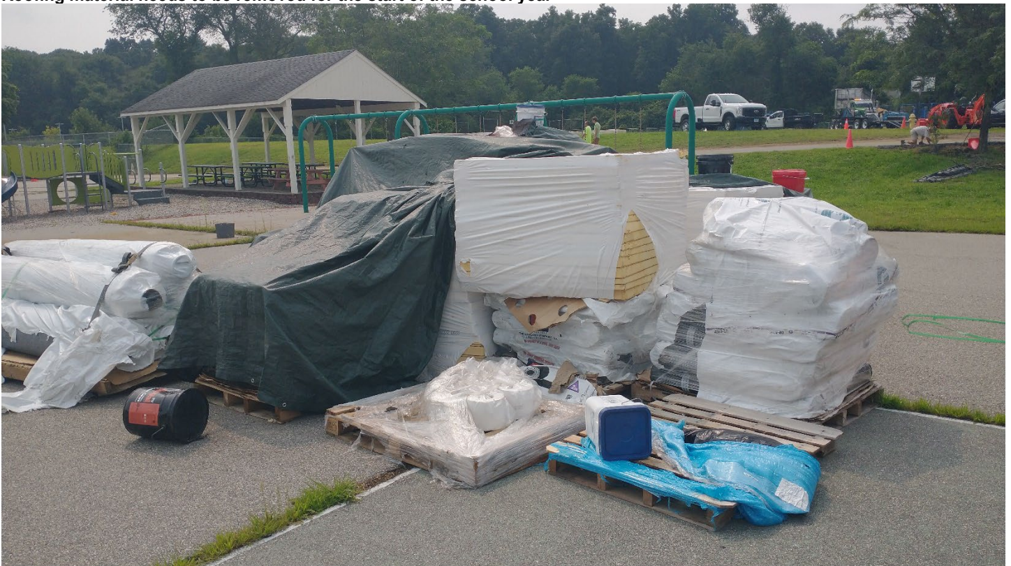
Roofing material needs to be removed for the start of the school year
