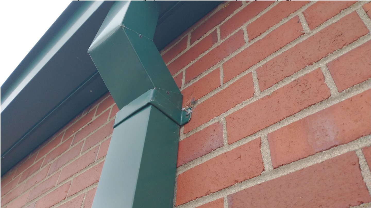
Roof A – Rivets for downspouts – Mandrel head (pin) needs to be flush with the primary head (ring)
