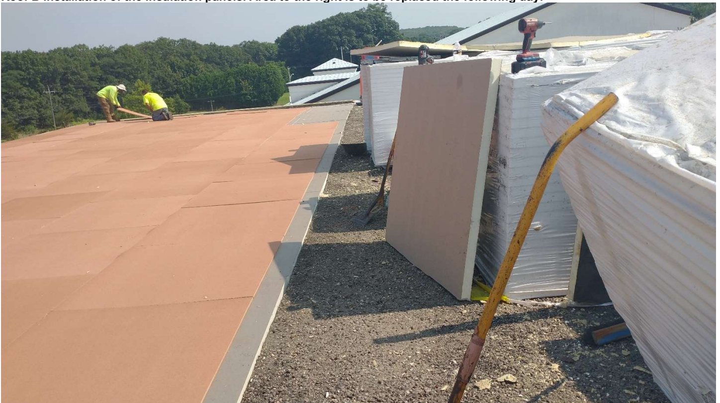
Roof B installation of the insulation panels. Area to the right is to be replaced the following day.
