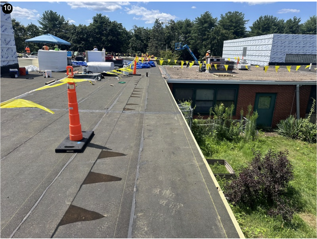
10 Field- Good bleed out at lap seams- Sheets lapped correctly for slope- Fascia blocking installed
