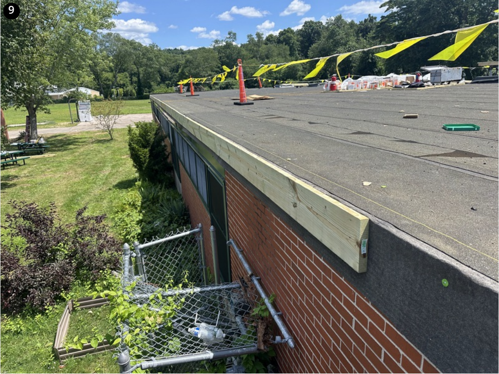
9 Fascia blocking has been installed around the perimeter-Will be covered with ice and water
