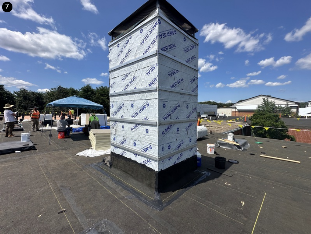
7 Chimney with completed ice and water application- Hat channels are secured- Base flashings completed with cant strips in place
