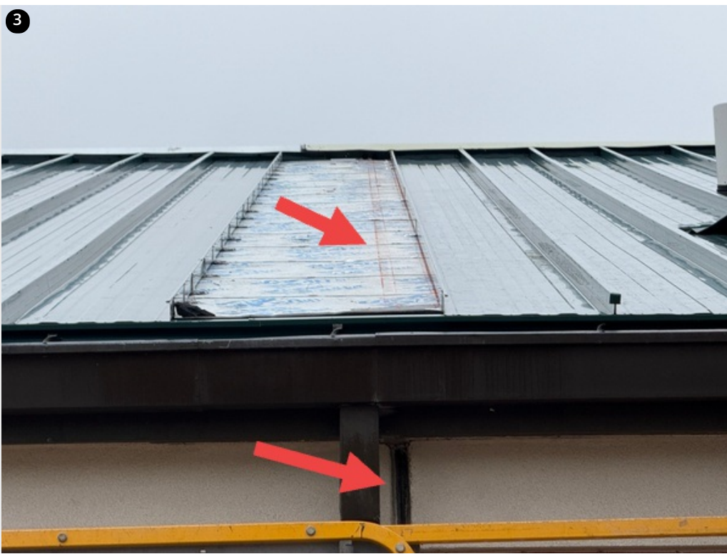
Expansion joint chalked out- 1/6/25
