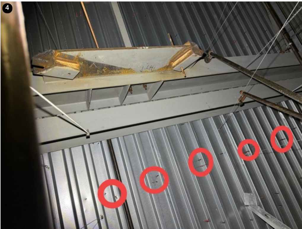
Fasteners observed penetrating deck- 1/6/25
