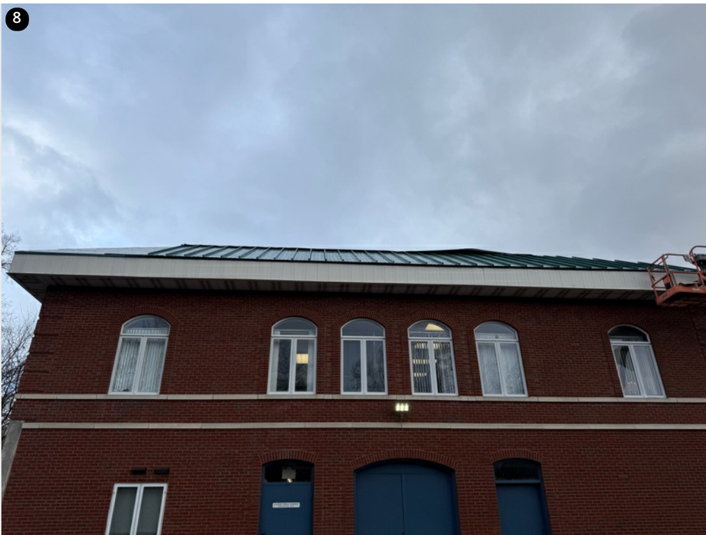
Panels are straight and free of camber- 11/22/24
