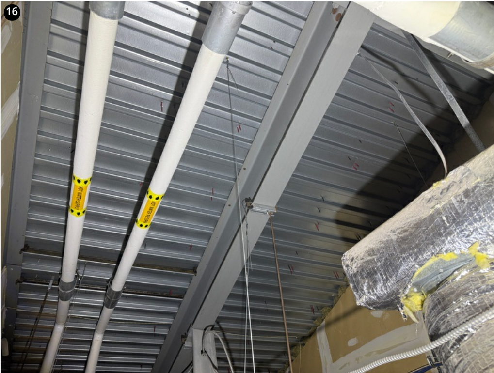
Fasteners observed penetrating deck- 11/27/24
