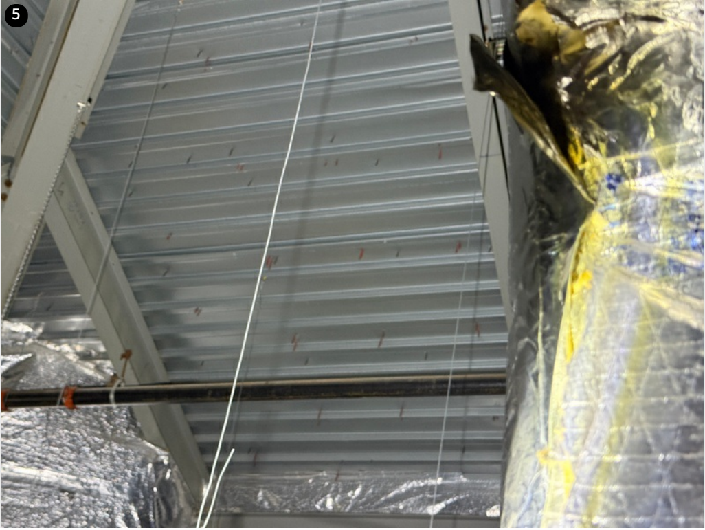
5 Fasteners observed penetrating deck- 11/23/24
