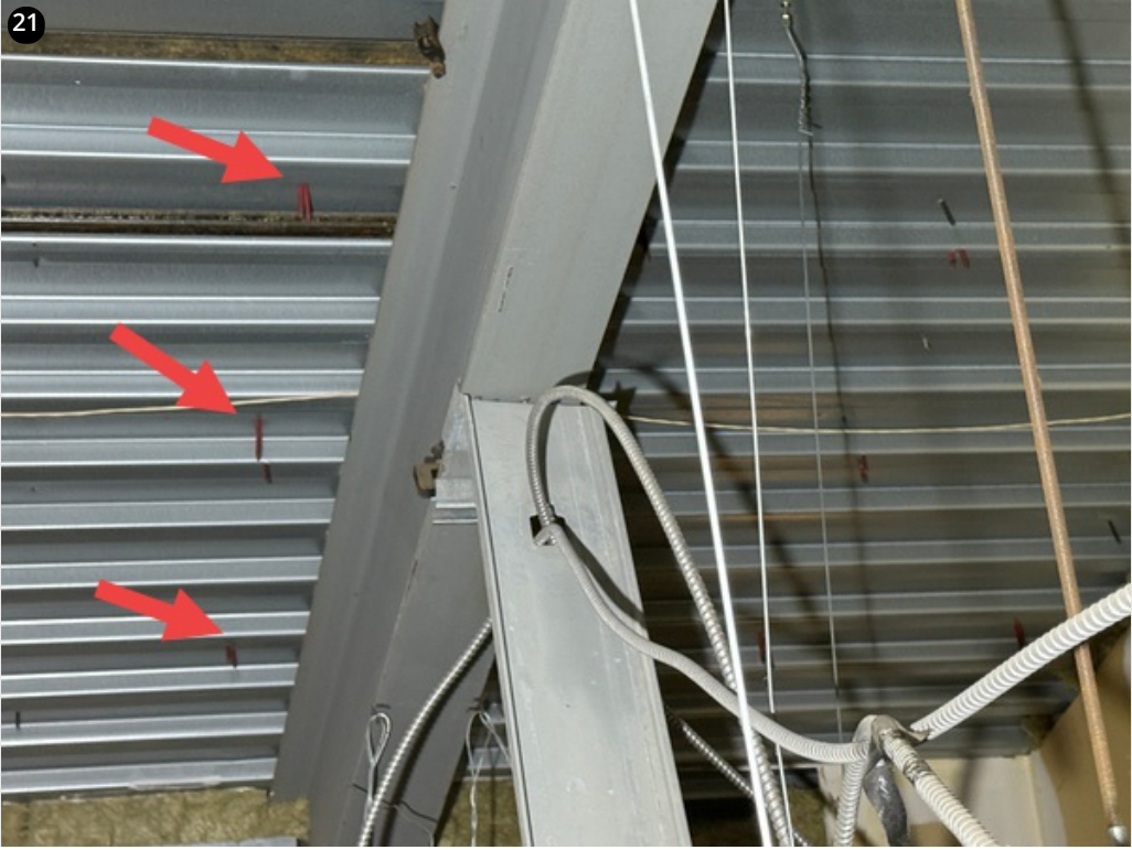
Fasteners observed penetrating deck- 11/29/24
