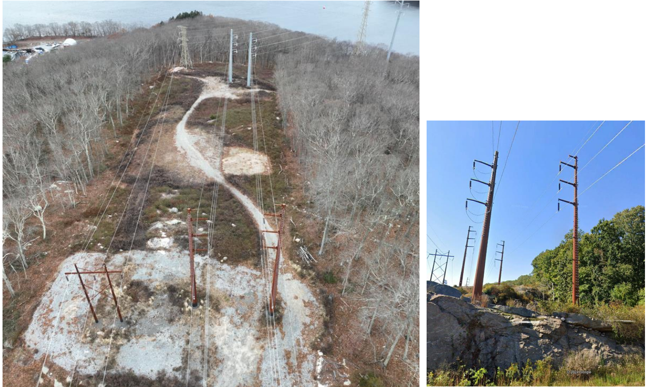
Figure 5. Eversource steel support structures adjacent to planned blasting that will take place to the right in each photograph.
