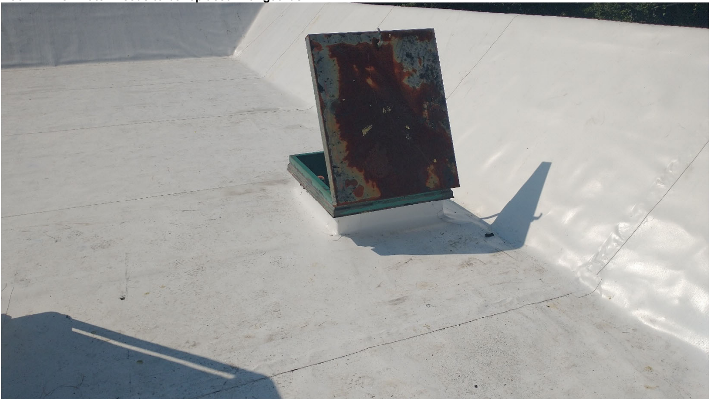
Roof B – New hatch needs to be replaced with guards
