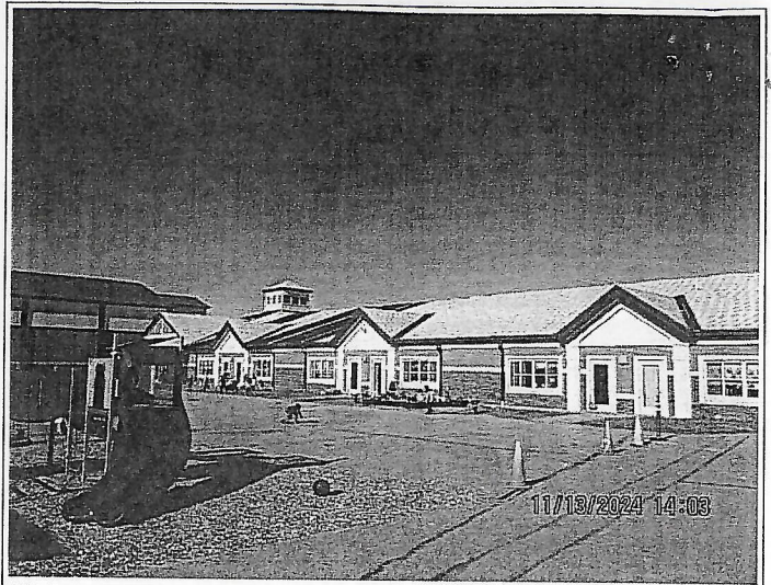
20. Underlayment have been installed on the entire substrate in compliance with the approved shop drawings.
