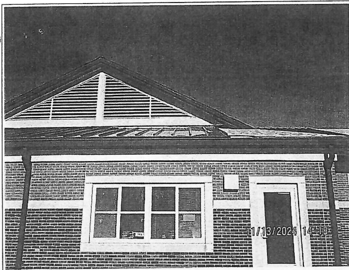
13. Dormer on back of main building. Panels are pan ended in compliance with shop drawings. Headwall flashing will be tucked under existing flashing, lined with a continuous bead of sealant and riveted with stainless steel, closed end rivets at 4" oc..
