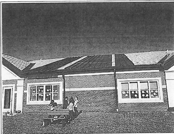
2. Staged panels have one screw securing them to the roof and are tied down. These panels are not considered installed. Staged panels should be installed as soon as possible as this may cause an unsafe condition.
