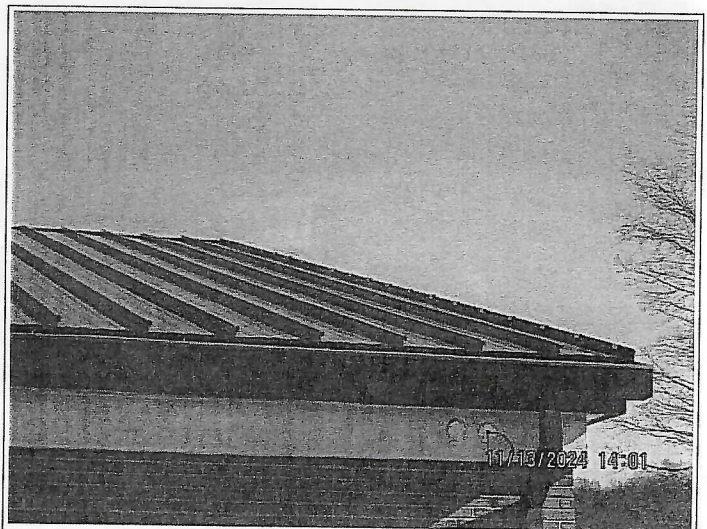
12. Same location. Gable clips must be installed at 17" in the 8' high pressure zone in the upper right corner. The remain gable clips are to be spaced at 20". Refer to the approved shop drawings.
