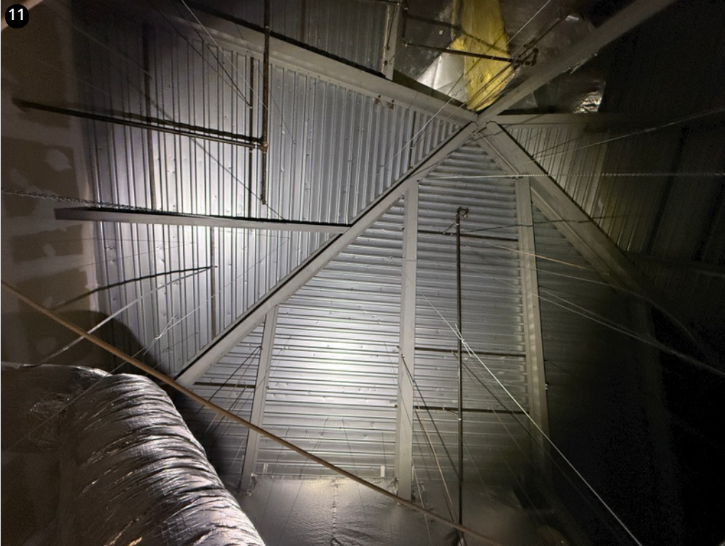
11 Fasteners seen through deck- 11/14/24
