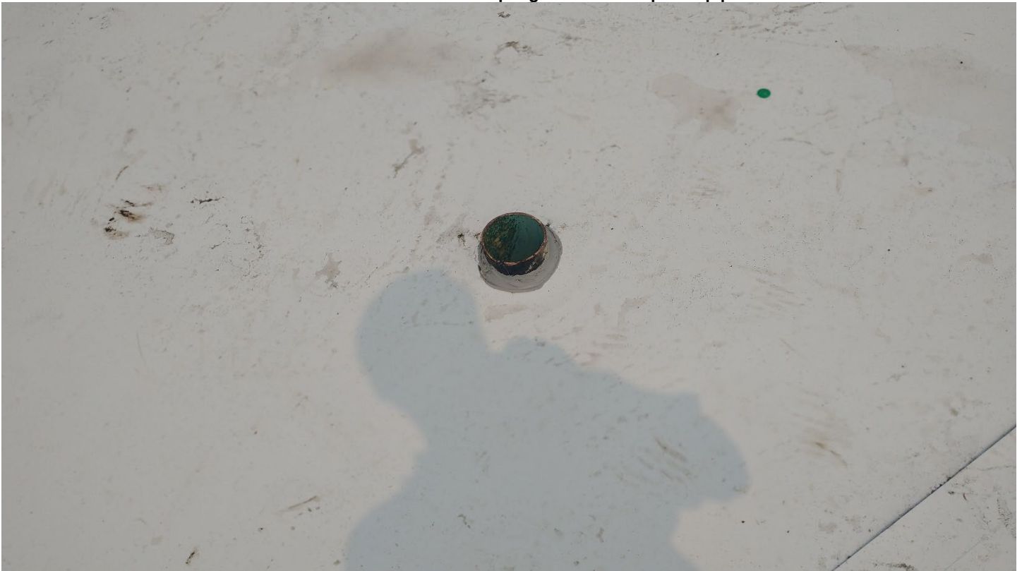
Roof A – Roof vent sides are too short will insert an inner coupling to hold the top vent pipe to the lower
