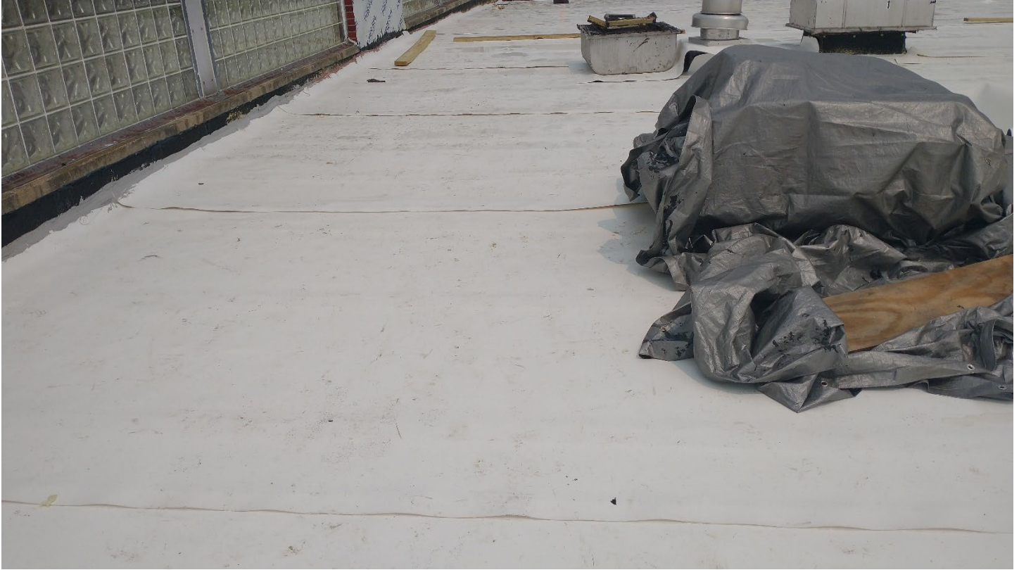
Roof A – Seams need to be welded
