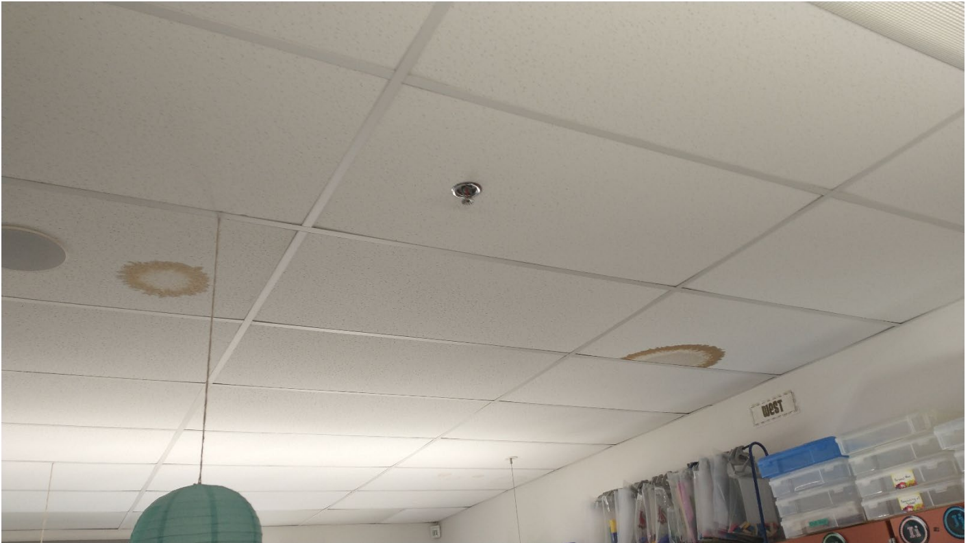
Room 227 roof leaks
