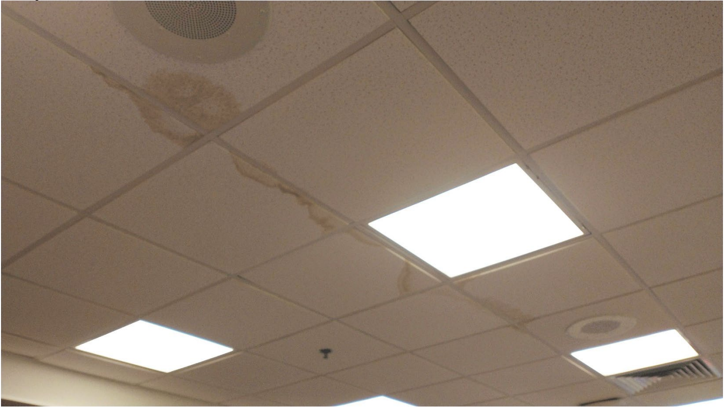
Library roof leaks
