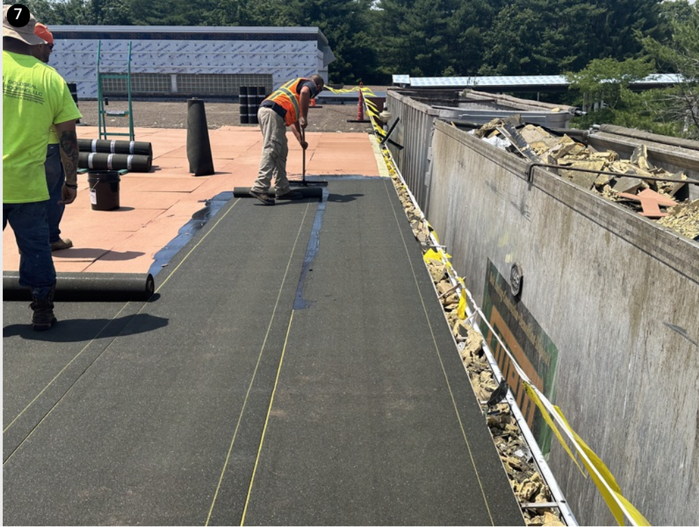
Crew rolling base sheets out over insulation and cover board using cold adhesive
