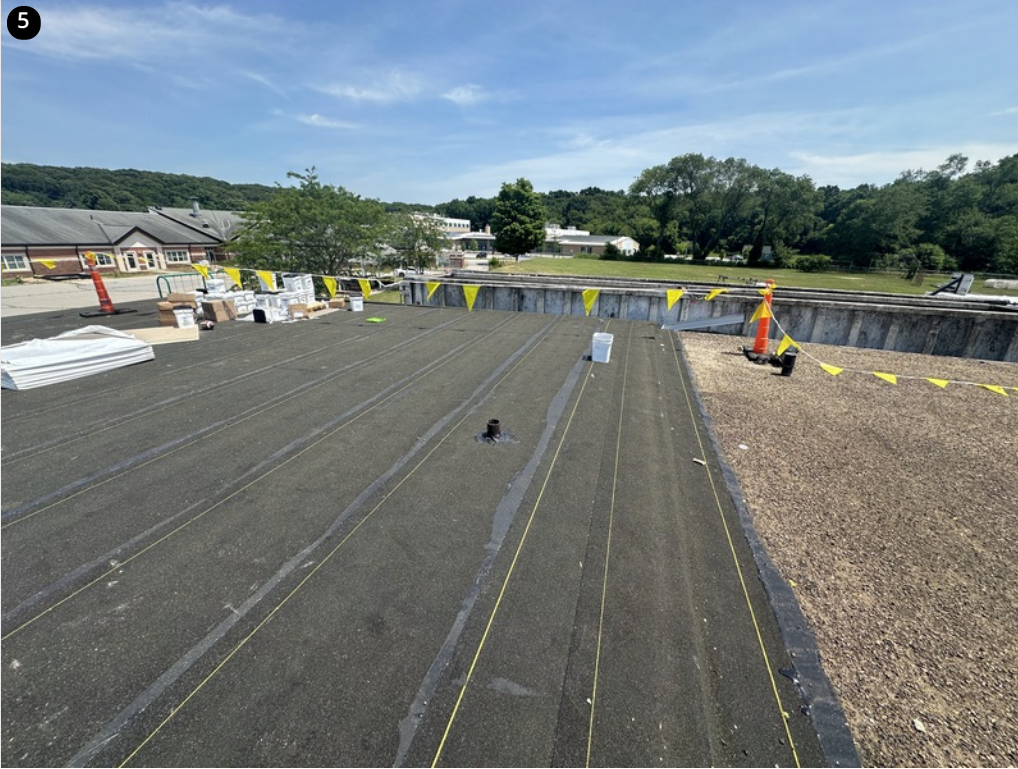
Base sheets installed over insulation and coverboard- Good bleed out at lap seams
