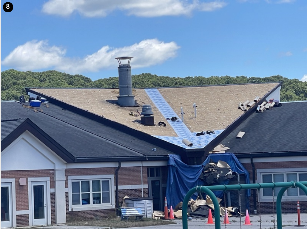
8 Valley section ripped to deck- Valley reinforced with ice and water layer
