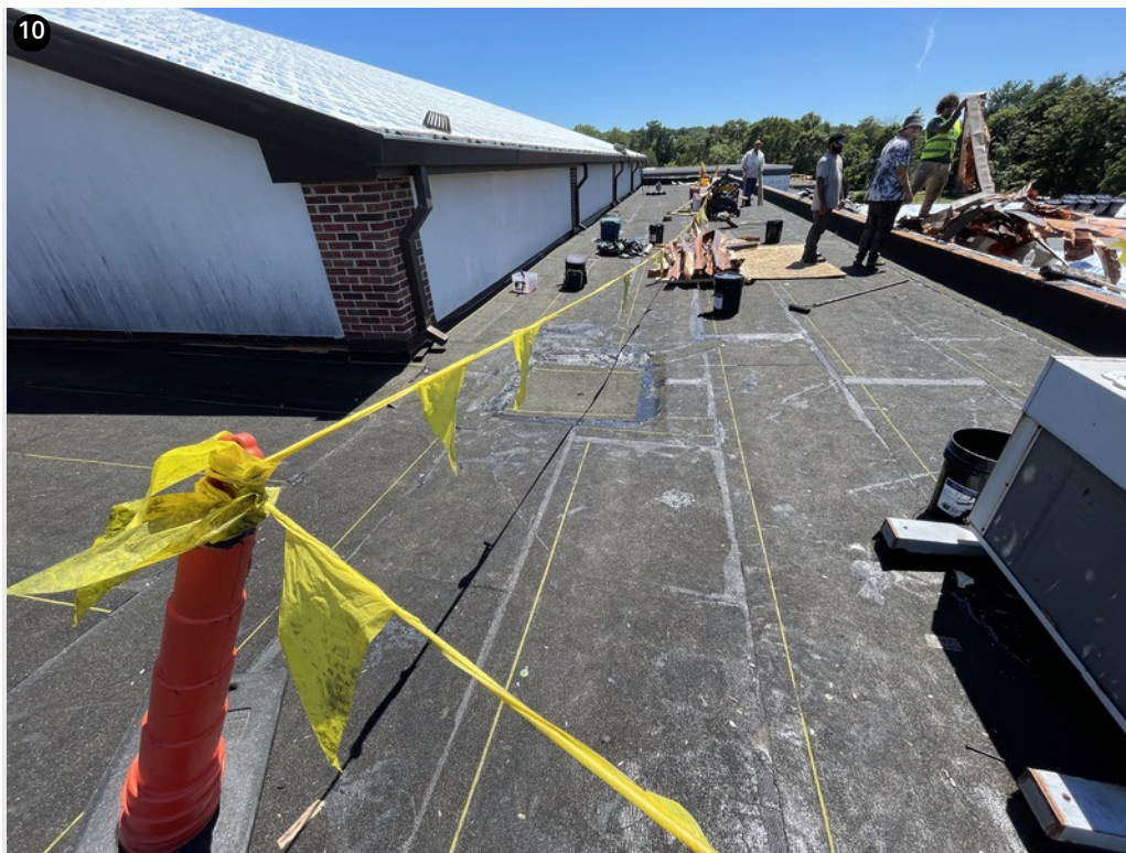
10 Low slope roof section base sheet is completed and drains are temped in
