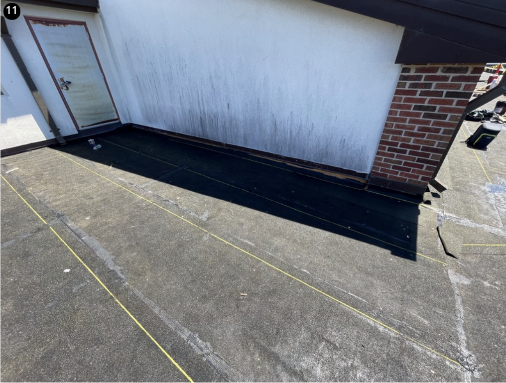
The crew will install the base sheet flashings prior to the cap sheet
