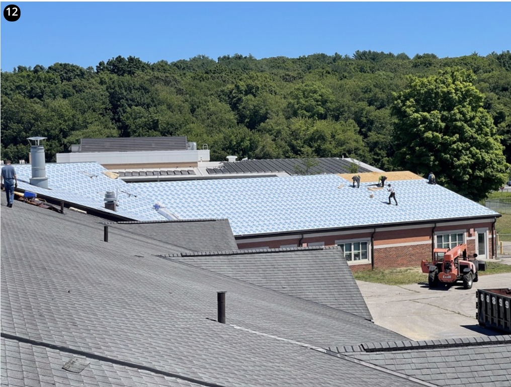
The shingle crew ripped the furthest interior section and finished the valley
