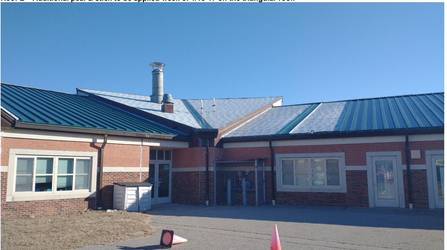
Roof E – Additional peel & stick to be applied week of 1/13-17 on the triangular roof.
