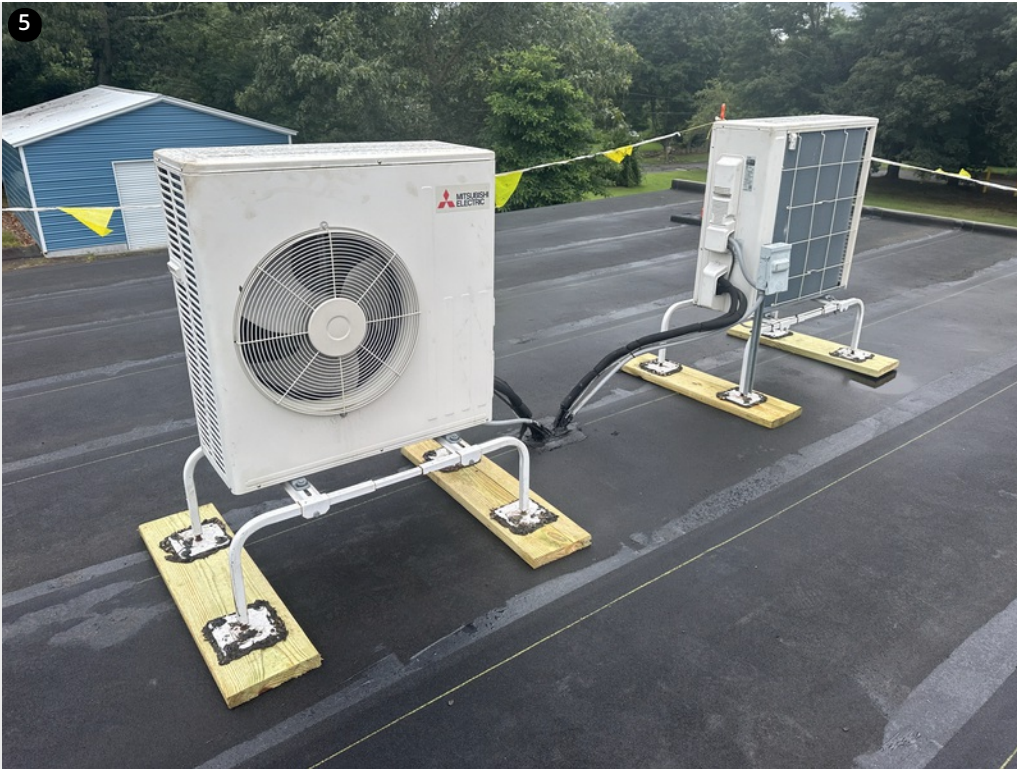
Split units on new sleepers- Previously fastened directly through flood layer of roof- Cause of consistent leaks
