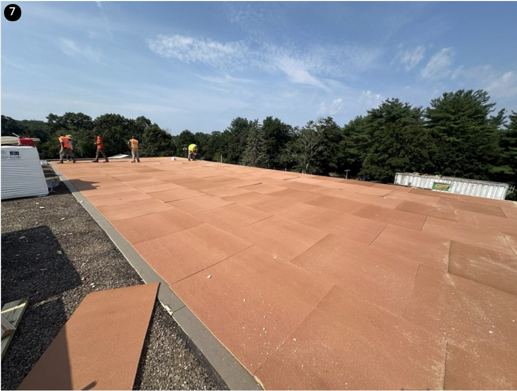
Upper roof section ripped to deck- 5" of insulation and coverboards being installed
