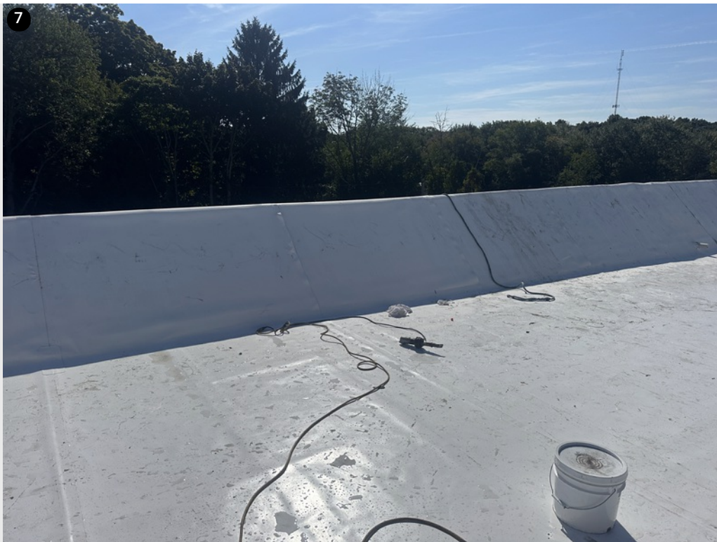
7 Overview- East wall with cap sheet installed- Crew heat welding vertical seams
