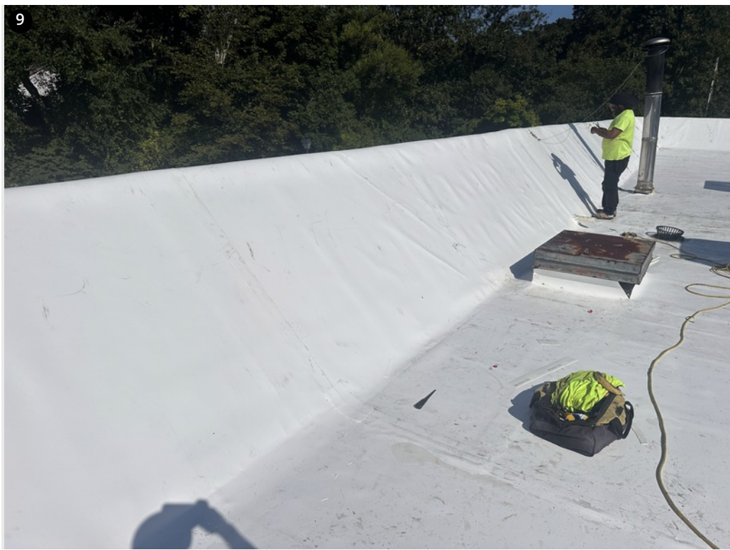
9 Overview- West wall near roof hatch- Roof hatch prepped for curb flashings
