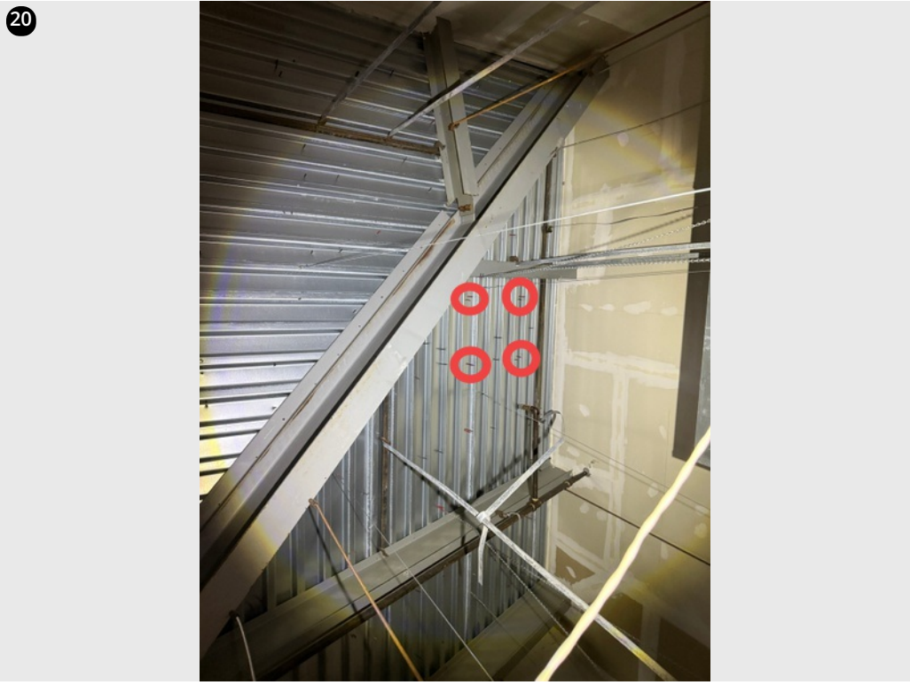
Fasteners observed penetrating deck- 12/14/24
