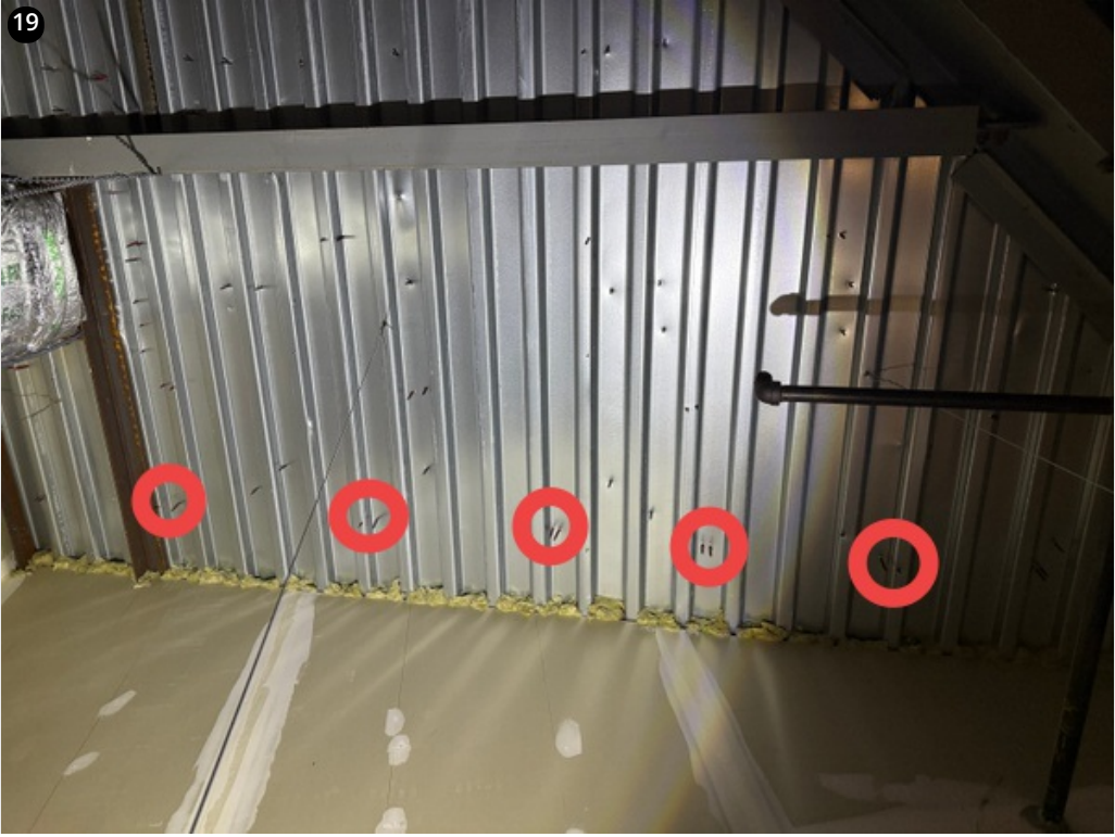
Fasteners observed penetrating deck- 12/14/24
