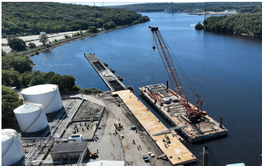
Newly constructed pier with Montville Power Plant and transmission lines in background
