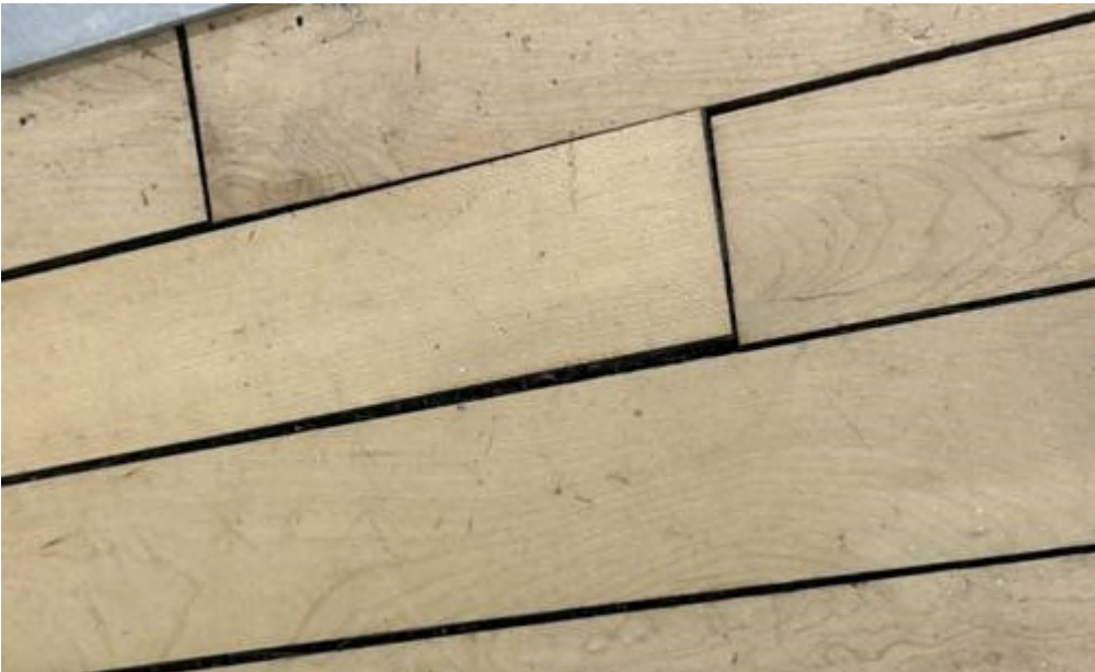
Floor boards separating and even breaking apart.
